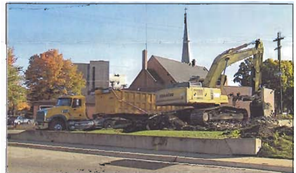
Photo (3): the heavy equipment is moving in to remove the house from its frame.
